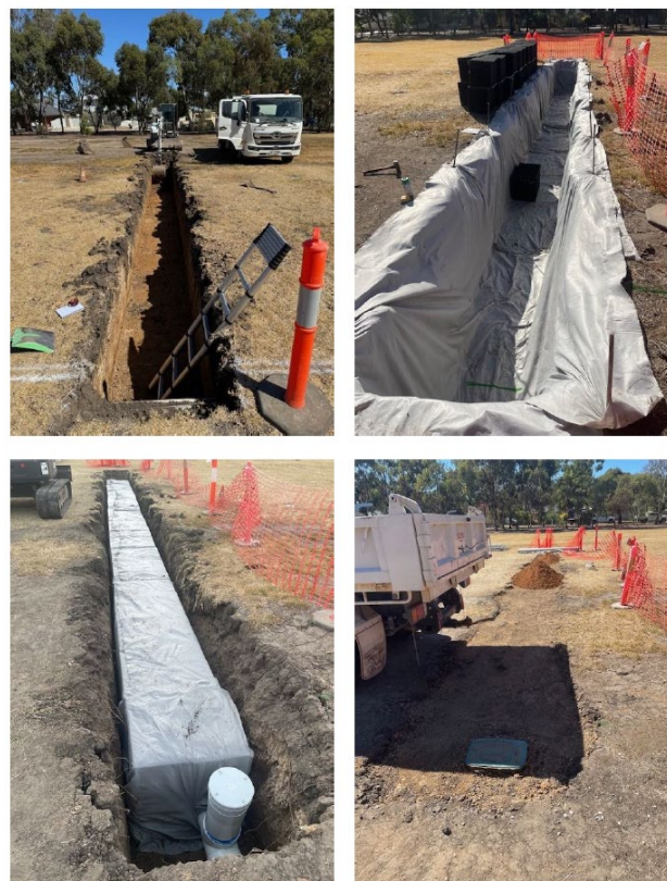
Figure 7: Soakage trench construction in St Marys Street Reserve in 2025 (Images: Rajibul Karim and Don Cameron)
